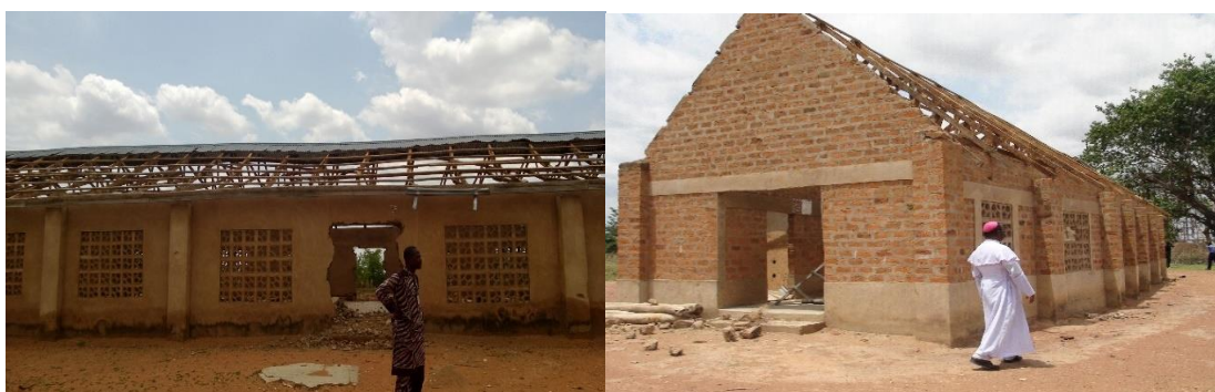
One of the Bishops inspecting vandalized churches (Source: NCSAN)
