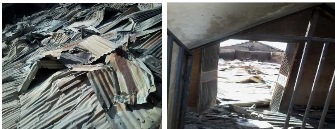
Burnt roofing sheets of one of the Evangelical Reformed Church of Christ at Yelwan-Bassa, Kokona LGA of Nasarawa state (Source: NCSAN)
